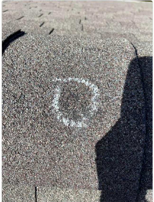
Chalk-circled hail hit on flat slope near wall-to-roof transition shows granule loss exposing mat substrate.
