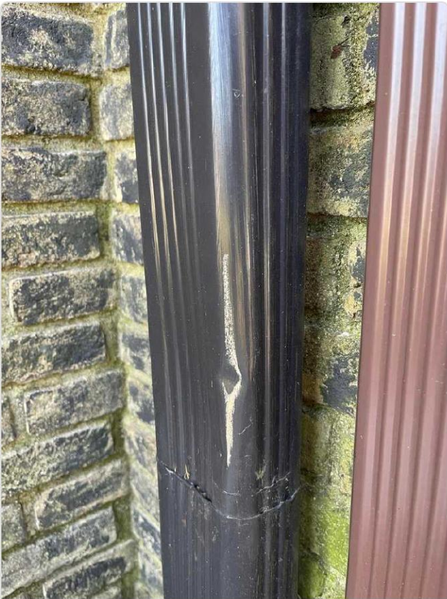
Chalk test on black aluminum downspout reveals circular gap confirming hail dent impact.
