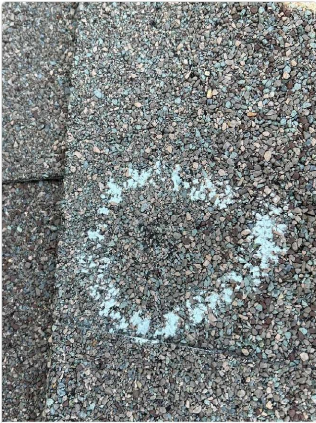
Chalk-circled hail strikes on flat slope near skylight — granule displacement confirms mat fracture.
