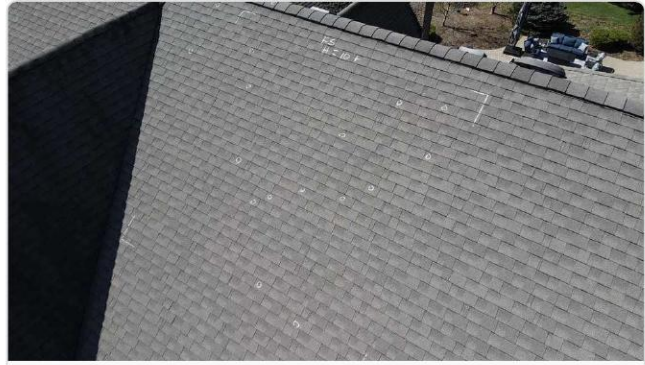
Front slope test square reads FS H=10; 20+ chalk-circled hail strikes across field confirm replacement threshold.
