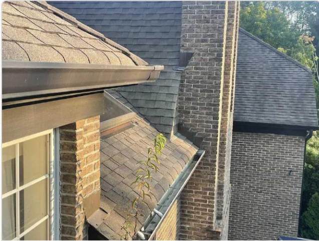
Wall-to-roof transition shows aged step flashing with plant growth in gutter — debris retention compounds storm vulnerability.
