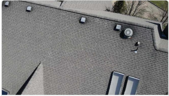
Aerial overview shows chalk-marked test squares with hail hit counts across rear slope and ridge.
