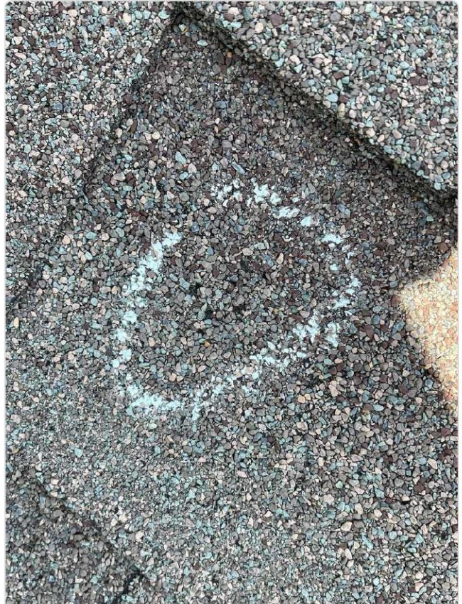
Chalk-circled hail strike on shingle shows granule loss exposing dark asphalt mat — confirmed impact fracture.
