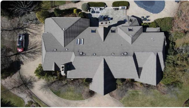
Aerial overview of complex roof with 7+ skylights, multiple valleys, and numerous penetrations requiring full replacement.
