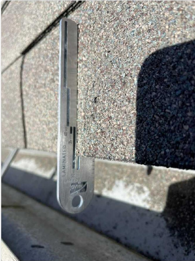
HAAG hail gauge on laminated shingle measuring impact diameter — professional damage documentation.
