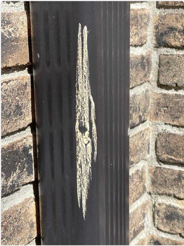
Chalk test on aluminum downspout reveals circular gaps in chalk line confirming multiple hail dent impacts.
