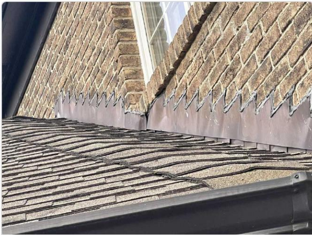
Step flashing at brick wall shows severe distortion and lifting; shingle courses along transition exhibit hail damage.
