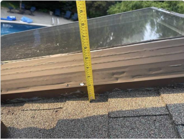
Tape measure shows skylight curb height ~5 inches; hail dents visible on aluminum frame flashing.
