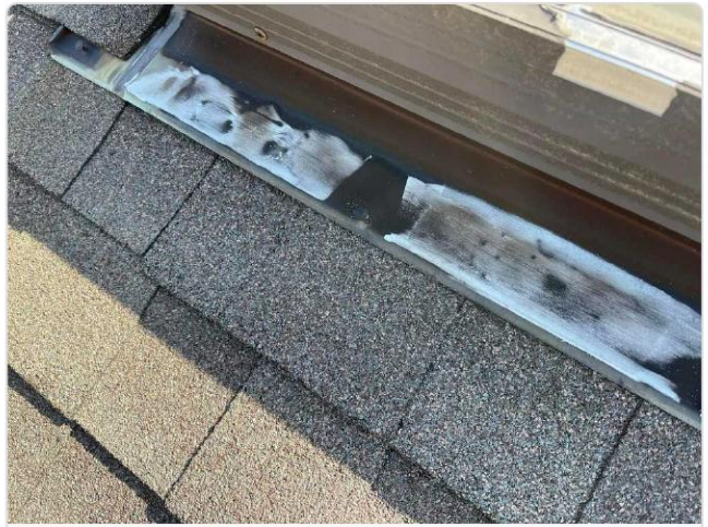
Skylight base flashing shows deteriorated sealant and hail dents on metal apron flashing.
