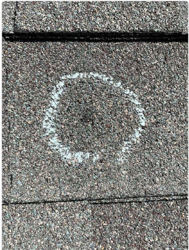
Chalk-circled hail strike on shingle exposes displaced granules and dark asphalt mat.
