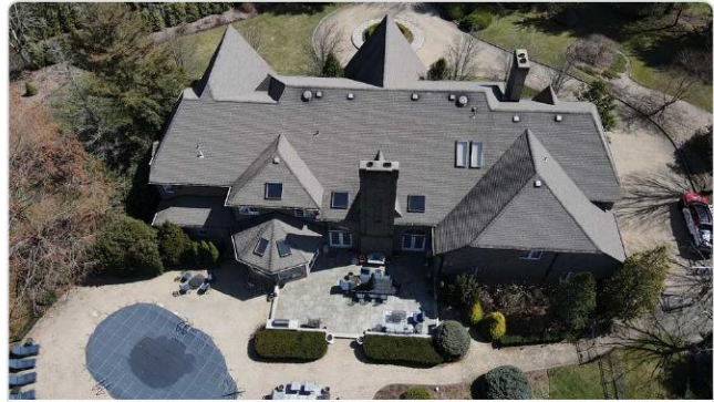
Aerial overview reveals complex roof with 7 skylights, multiple valleys, and copper flashings requiring full replacement.
