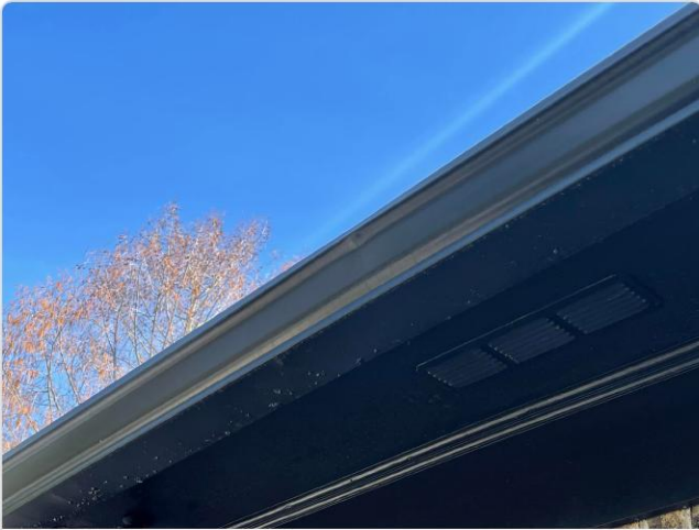
Dark aluminum gutter and soffit vent from below; no chalk test visible but soft metal is candidate for hail dents.
