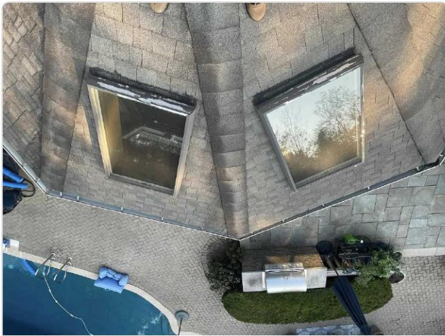
Aerial overview shows complex roof with dual skylights, multiple valleys, and hail-vulnerable copper flashings over pool area.
