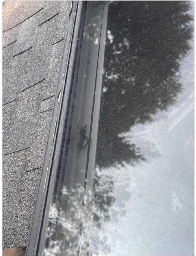
Skylight frame and flashing detail — shingle courses show wind creasing adjacent to skylight edge.
