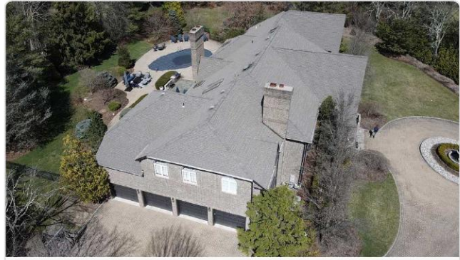
Aerial overview of full property showing complex roof with multiple slopes, 7 skylights, and two chimneys.
