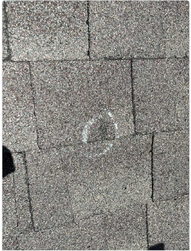
Chalk-circled hail strike on laminated shingle shows granule displacement exposing dark mat — confirmed hail damage.
