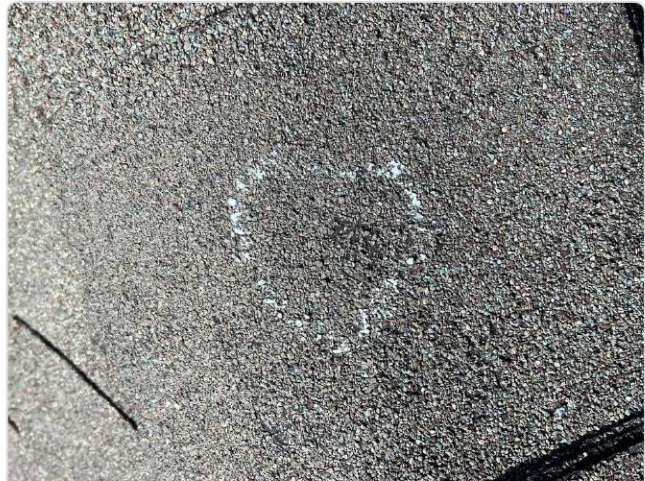
Chalk-circled hail impact on shingle surface with granule displacement — mat fracture confirmed.
