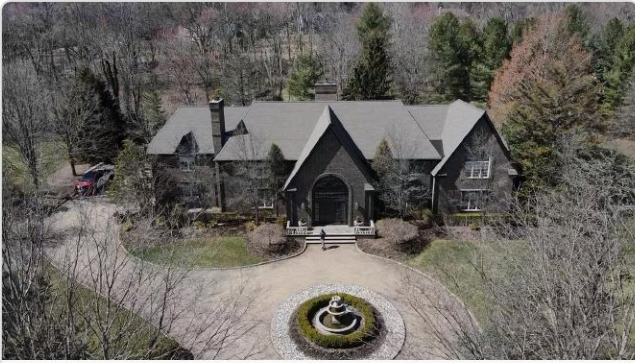
Aerial overview of estate roofline shows complex geometry with 7+ skylights and multiple ridges requiring full replacement.
