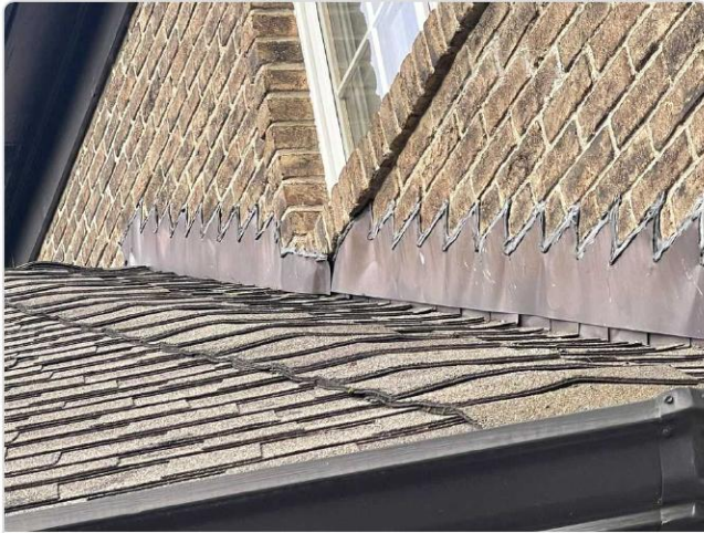
Step flashing at brick wall shows severe distortion and lifting; shingle courses along transition exhibit hail damage.
