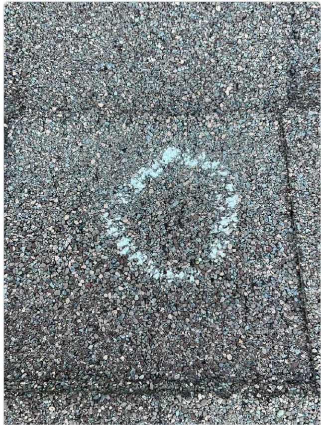
Chalk-circled hail strike on shingle shows granule displacement exposing dark asphalt mat — confirmed hail impact.
