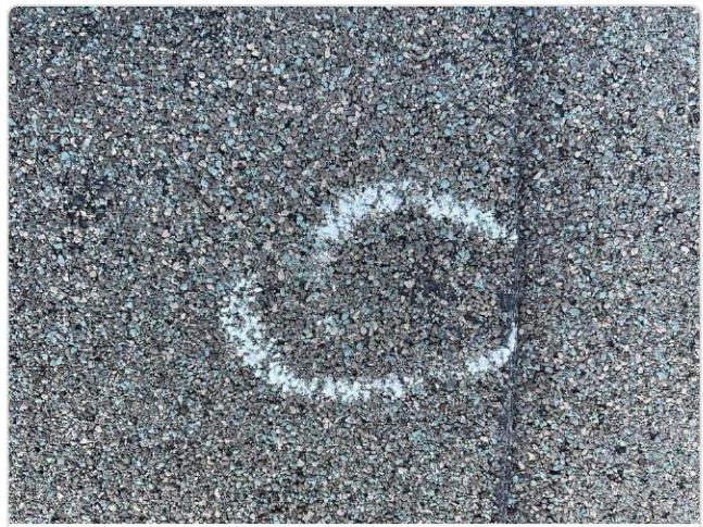
Chalk-circled hail impact on flat slope confirms repeatable dent pattern with granule displacement.
