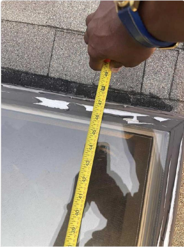
Skylight frame measured at ~49 inches; flashing sealant deterioration and hail-exposed edges visible at top rail.
