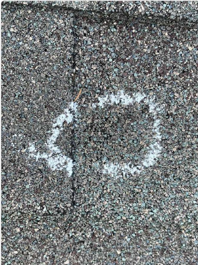
Chalk-circled hail strike on shingle shows granule loss and mat fracture at impact point.
