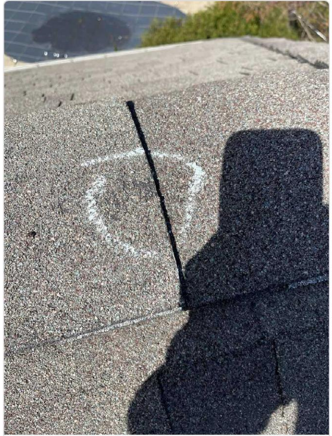
Close-up chalk-circled hail strike on shingle shows granule displacement exposing dark mat — confirmed fracture.
